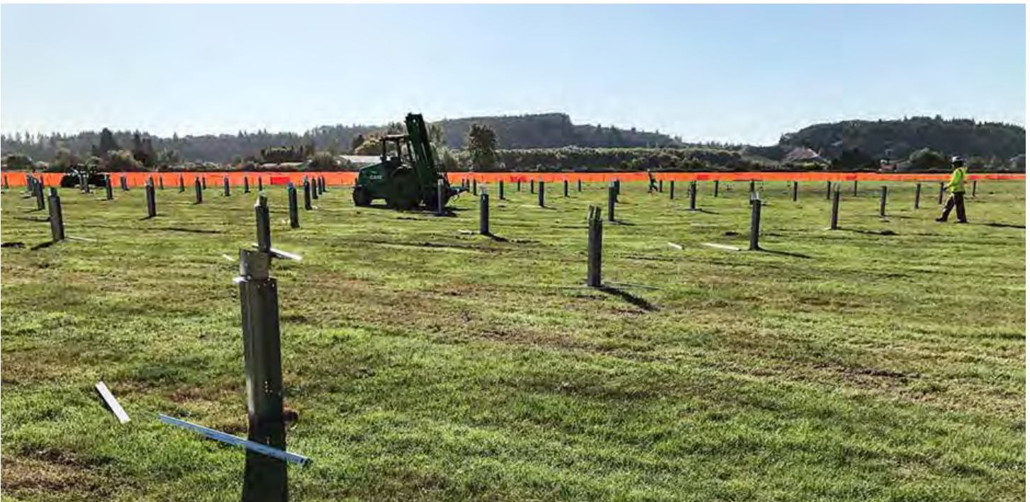
Solar site preparation and construction developed around existing vegetation, Photo by Jordan Macknick, InSPIRE project principal
